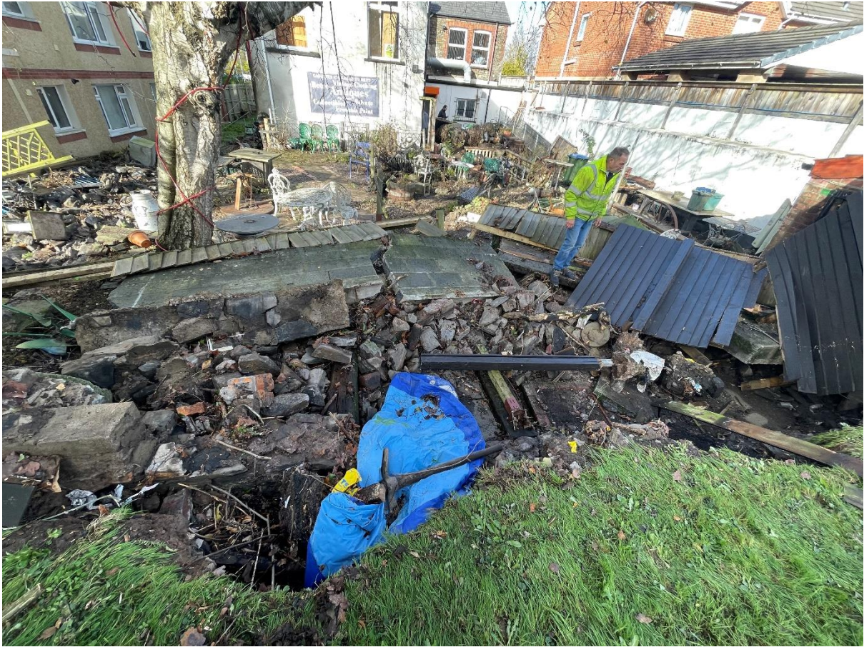
Figure 5 – Collapsed stone wall outside Vintage 7 Antique Centre.
