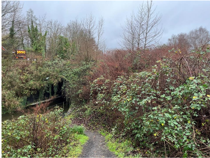
Photograph 9 – Knotweed on embankments – eastern Tennant Canal
