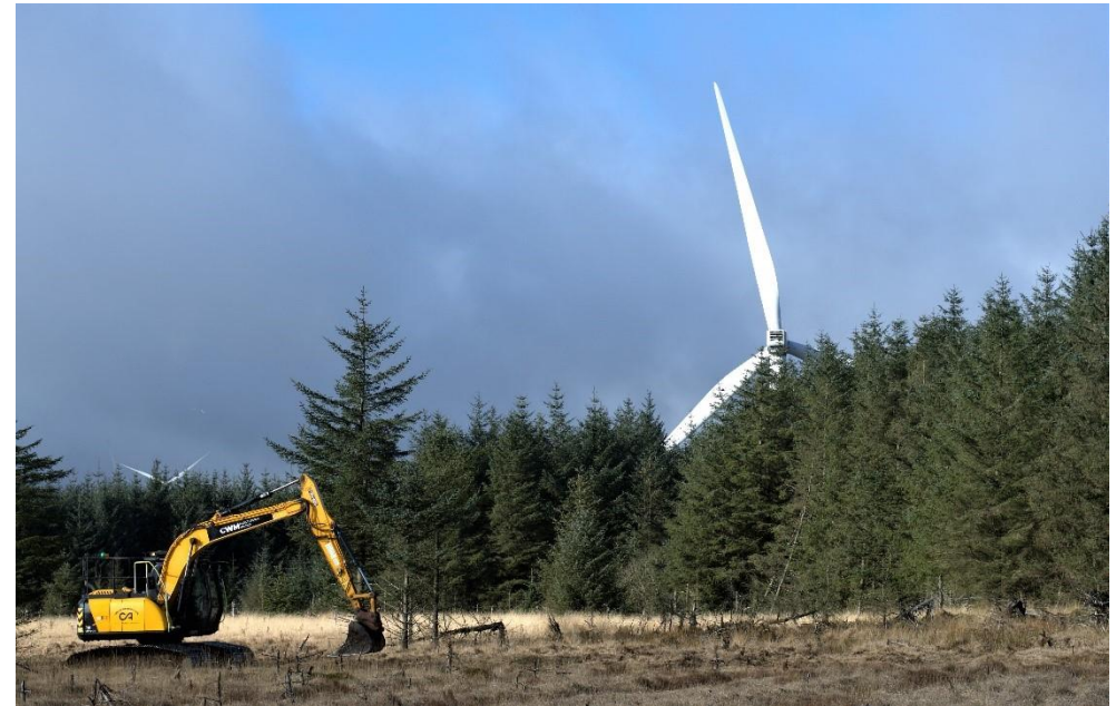
Figure 10: Castell Nos HRA - restoration in action. Excavators are modified to have wider tracks to reduce the risk of sinking
