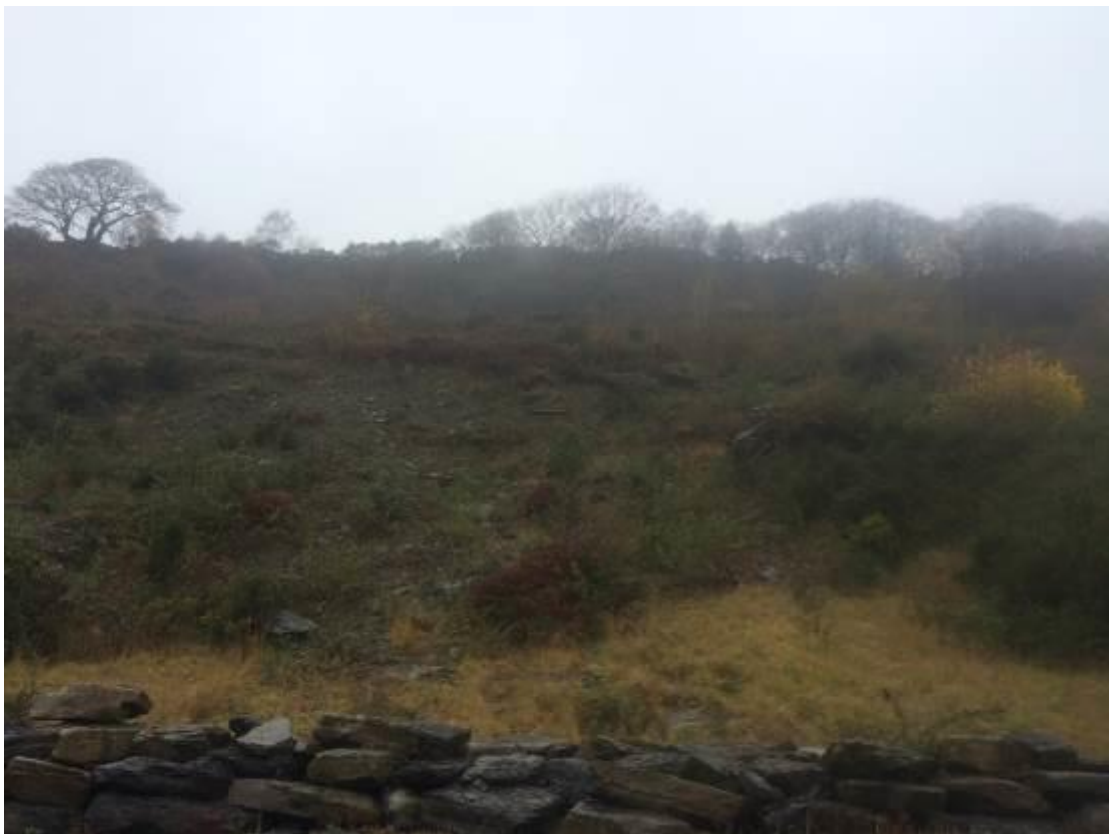
Photograph 20 – View of Panteg landslip with quarry beyond crest
